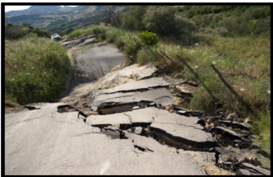
Broken road caused by earthquake.
