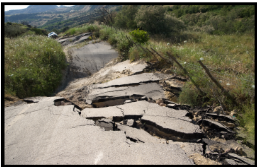
Broken road caused by earthquake.
